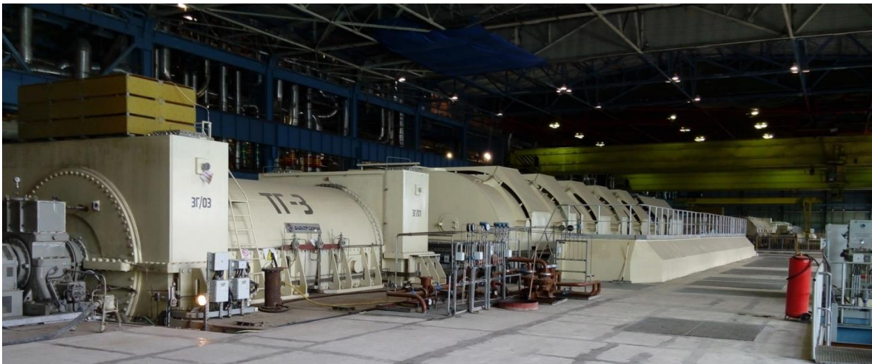
Turbine unit K-800-240-5
