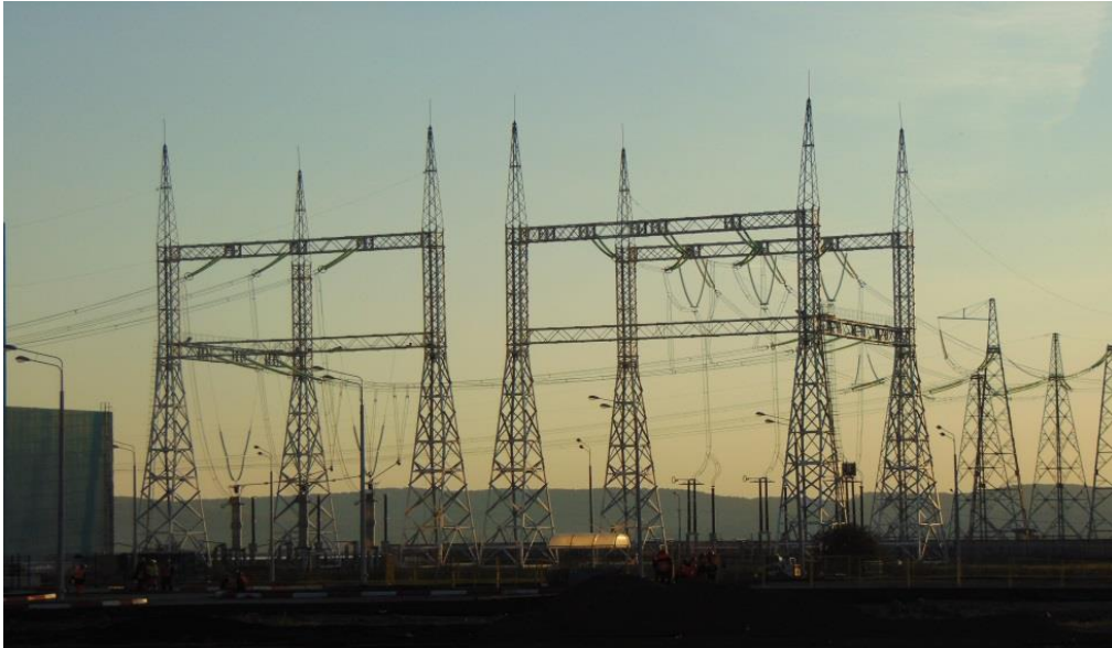
Busbar assembly (BA-2) - open switch yard - 500 kV
